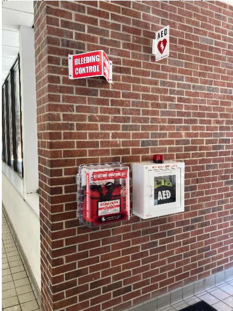
Figure 5: Stop the Bleed Trauma kits installed through City Facilities.
