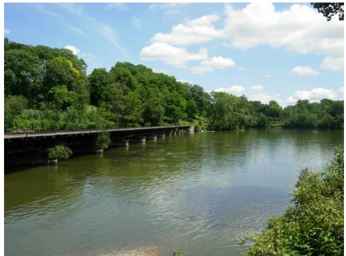
The abandoned trestle from the Industrial Flats toward the Foremost Dairy site
