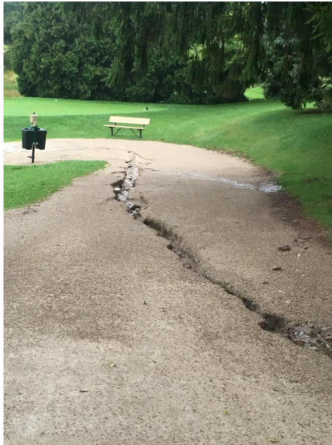
Cart path from #12 green leading to #13 tee washed out after a heavy rain.
