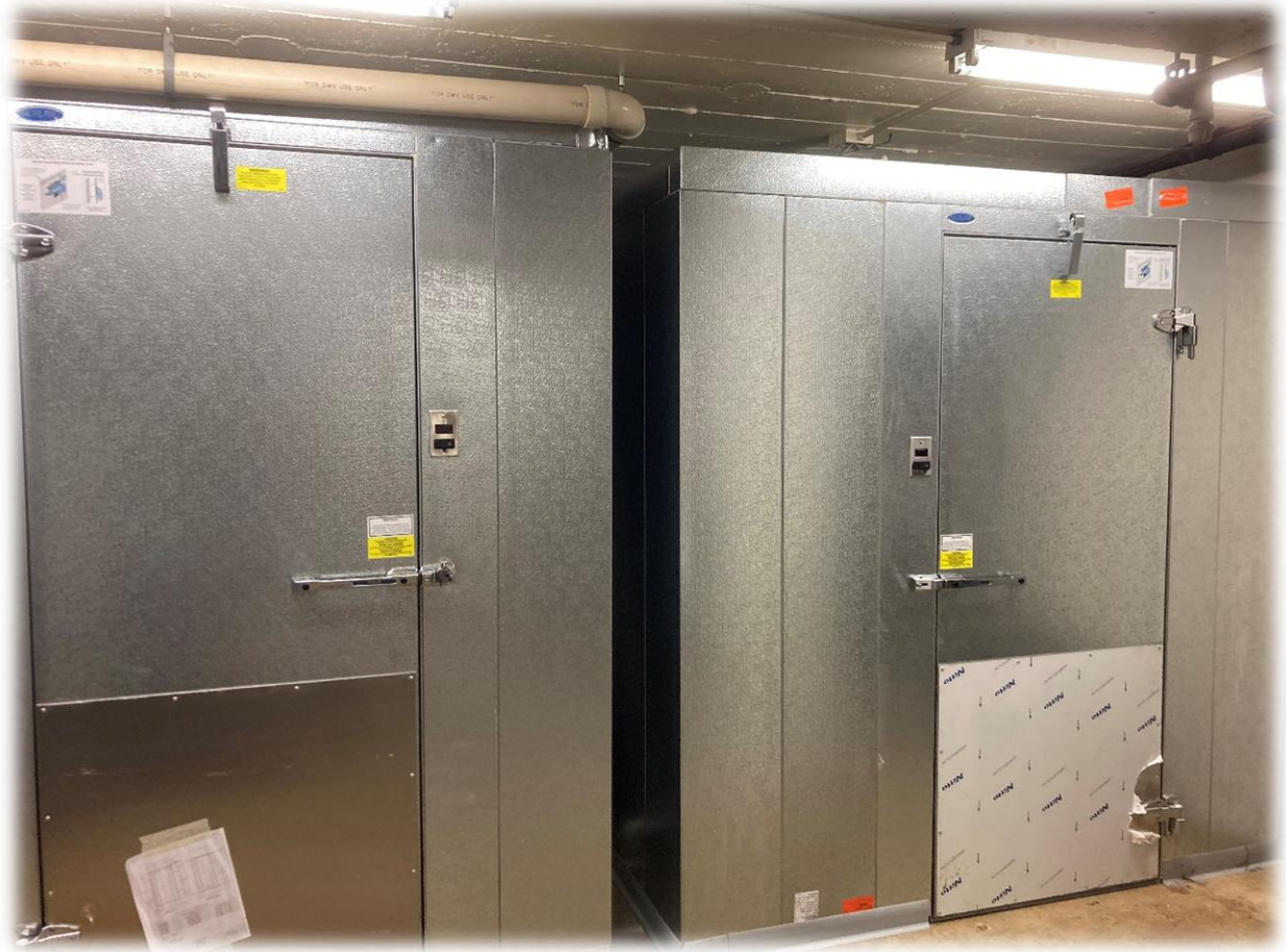
New units in the clubhouse basement, freezer on left cooler on right.
