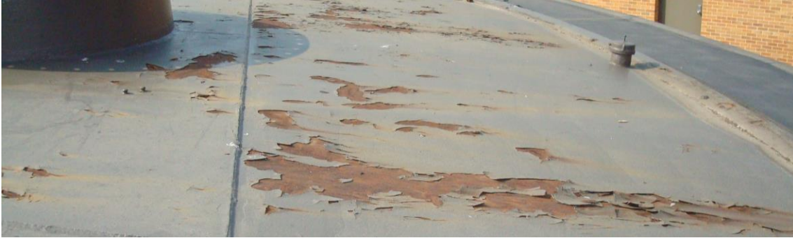
Photo #1: Secondary Digester #1 (West) Cover Depicting Severe Coating Failure.
