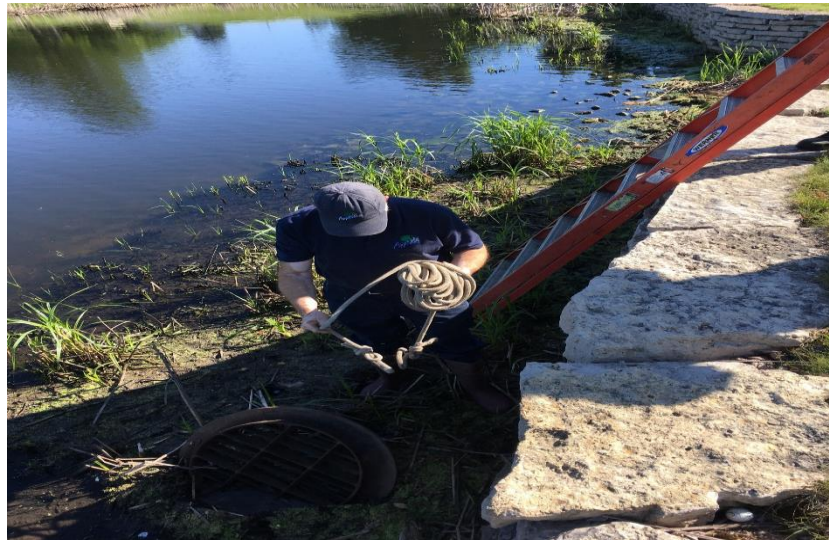
Jim Pedersen hooking up rope to pull catch basin lid from pond.
