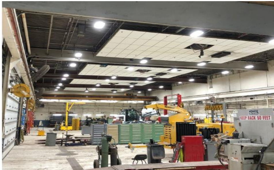
MSB CEA Mechanic Shop new LED fixtures installed
