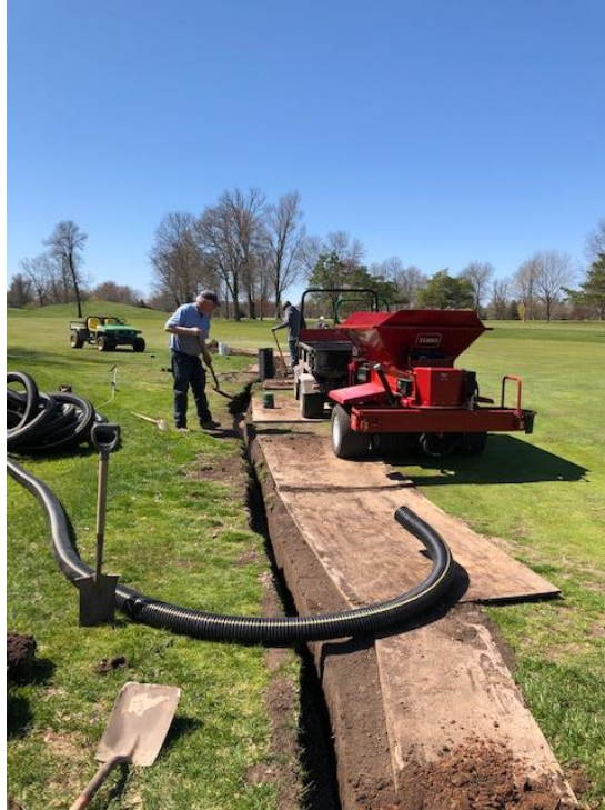
Utilizing the new topdresser/material hauler to back trench with pea gravel on #14.
