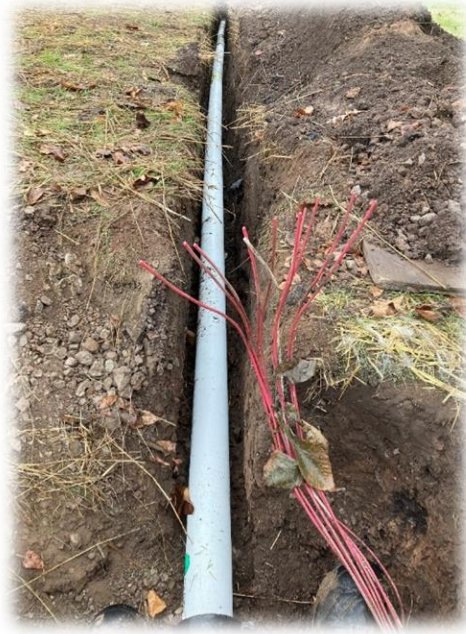
Rerouted irrigation along parking lot edge, irrigation wires needing to be spliced.
