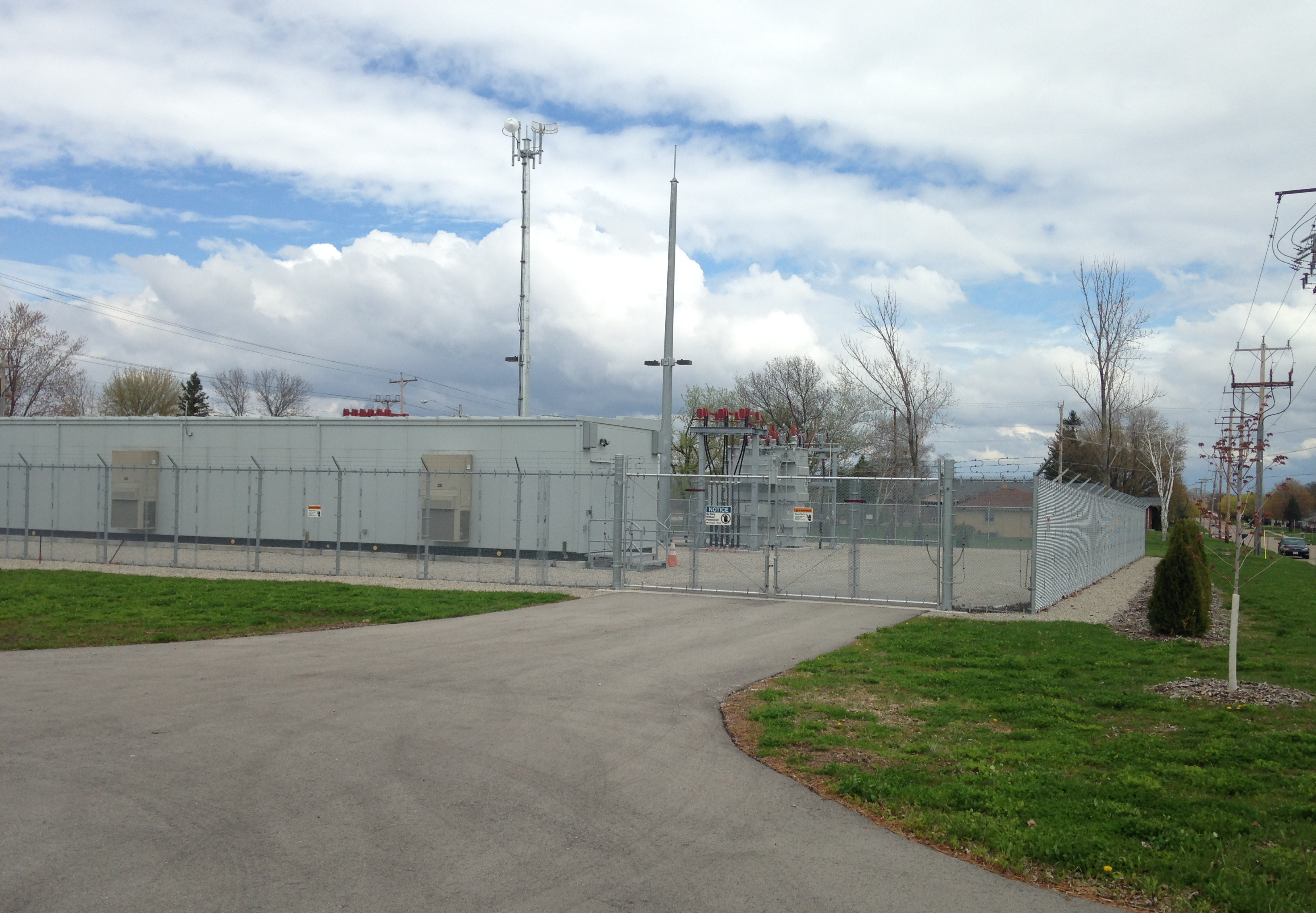
Example Substation Northland Substation from Southwest (Photo taken 05/01/17)
