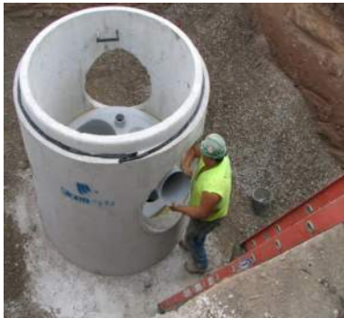
HSD's (Catch Basins)
