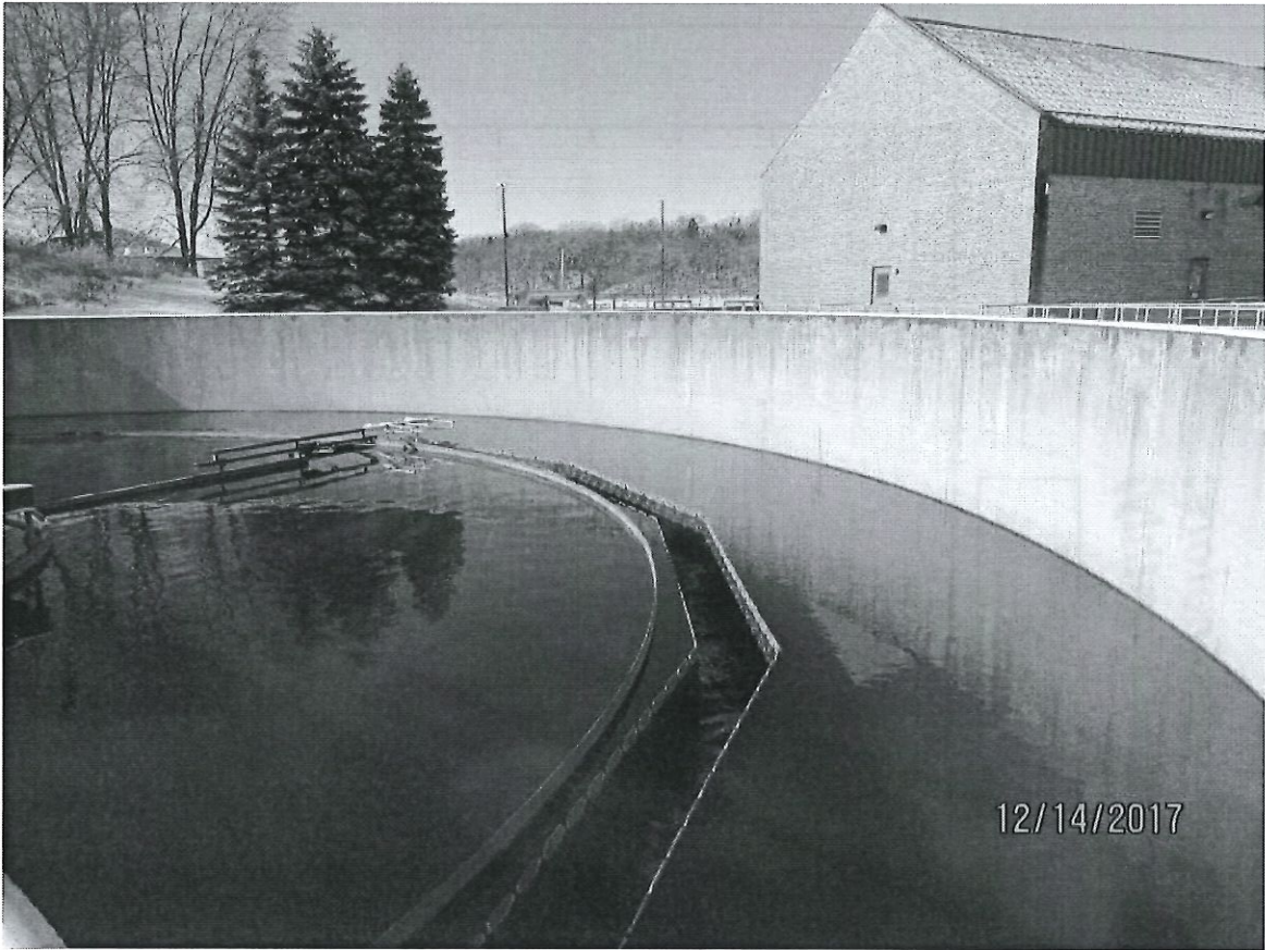
Close-up view of secondary clarifier
