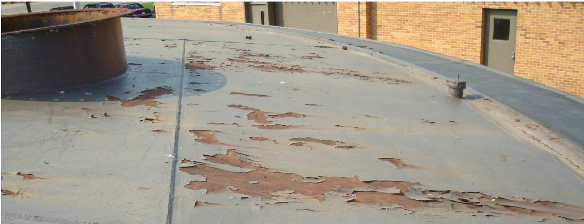
Photo #1: Secondary Digester #1 Cover Depicting Coating Failure.
