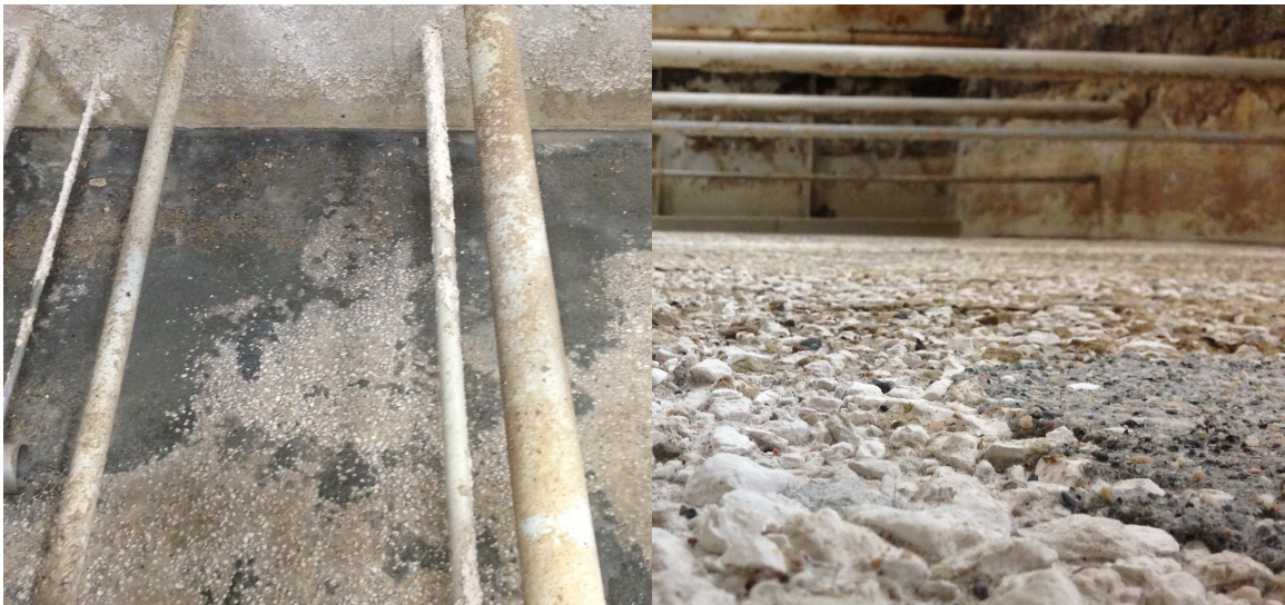
Photo 2: Receiving Station Tank #1 Concrete Deterioration
